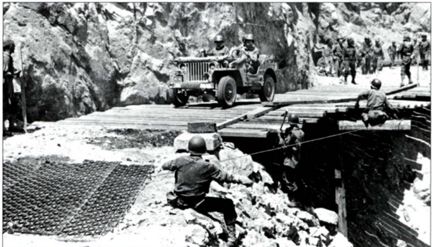
Members of the 10th Engineers, 3d Division build a temporary bridge to cover a hole blown in the roadway near Point Calava on the north coast of Sicily by retreating Axis forces, August 14, 1943.
