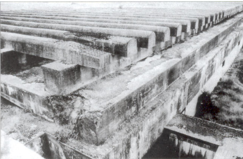
This photograph shows the so-called Fangrost bomb trap on the roof of the Bordeaux bunker. Concrete beams with a curved upper surface were laid over supporting square beams to create a space just above the roof of the bunker proper. Any bombs that hit the complex would detonate against these beams, with the blast being dissipated into the void. The system was highly successful, but had only been partially installed throughout the various bunker sites by the end of the war.
