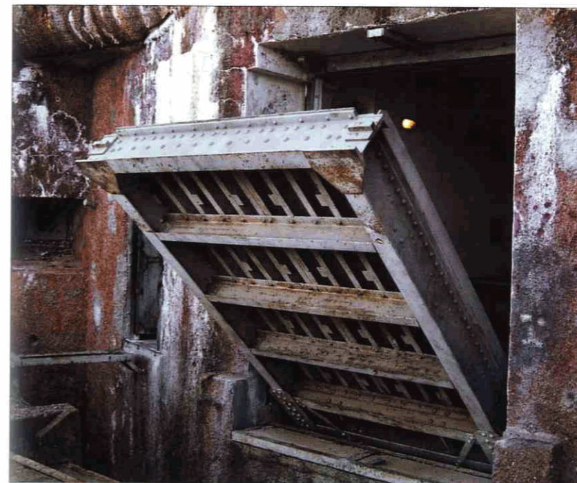
The entrance block of the gros ouvrage of L'Agaisen in the Maritime Alps. Its combination armoured door/drawbridge is in the half-raised position. Beyond the drawbridge, the garrison entrance door with its removable bridge and an automatic rifle embrasure are visible. (Author's photograph)
