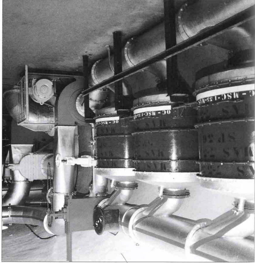
LEFT A portion of the primary filter and ventilation equipment in the support area of the gros ouvrage of Schoenenbourg. The large drums hold the air filters. Unfiltered air is forced into them from the ducts at the bottom by the fan in the background while filtered air exits from the top. (Marc Halter)
