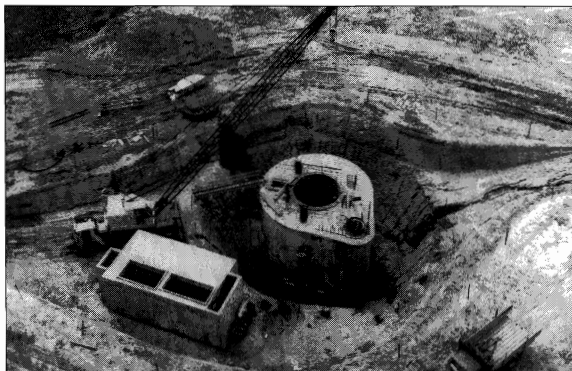
A Minuteman silo under construction near Ellsworth AFB, SD in June 1962. The launch support facility is to the left of the silo. (National Archives, Washington National Records Center, Suitland)
