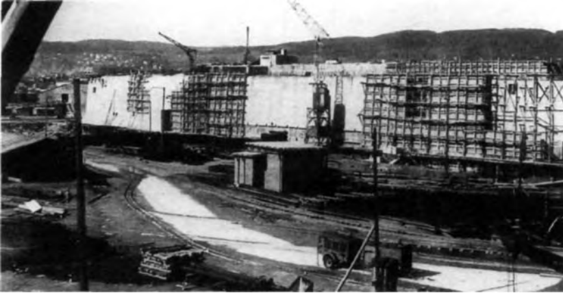
The Dora II bunker under construction. The construction of these bunkers required huge resources in men and materials, both of which were in short supply towards the end of the war, and hostilities ended before Dora II was completed.
