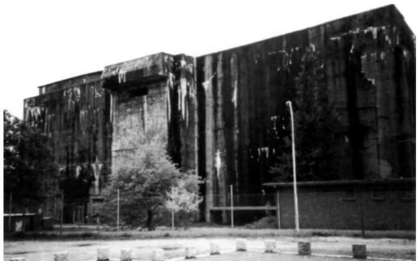
The Valentin bunker today. It is still used by the German military as a storage facility. The cost of demolition of such structures was astronomical so many were simply left standing and put to the most practical use possible.
