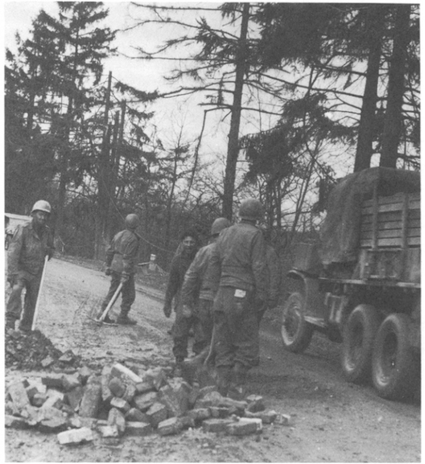
Co. C, 1st Combat Engineers repair shell damage to a road near Geyer, as a 2½-ton lorry passes. (US Army)
