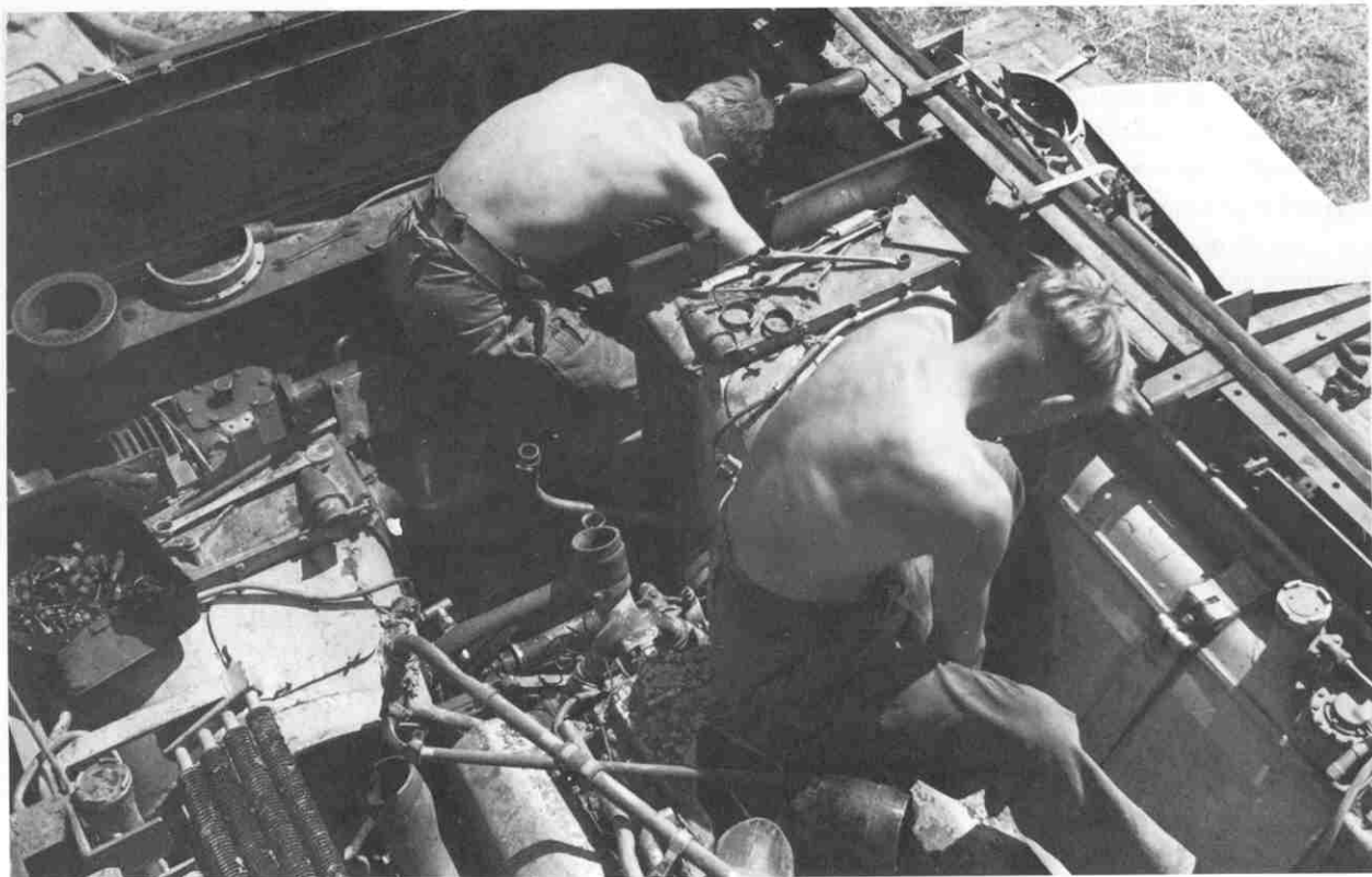
Fitters at work in the engine bay of a Cromwell. The nearest man is sitting on the Meteor engine with the left-hand fuel tank in front of him and the left-hand radiator to his left, while his mate sits on the gearbox to work on the final drive, steering and brake unit.
